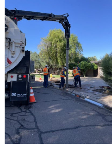
With so much complexity and so many pipes working to serve our community, water main breaks can happen anywhere and at any time.
