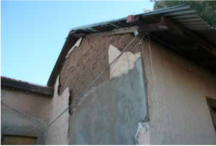
West Stucco Peel
