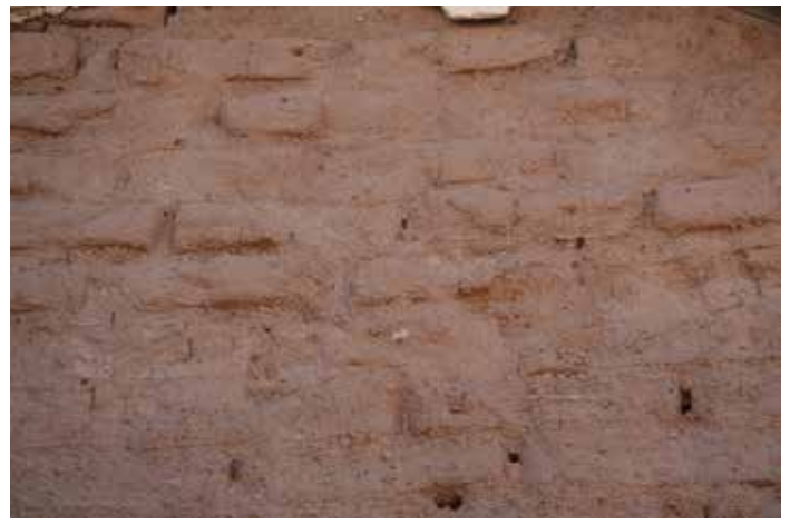
West Stucco Peel
