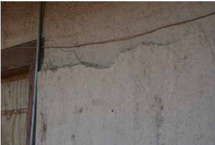
South Wall Buckling
