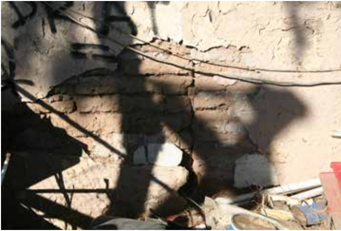
East Wall Damage
