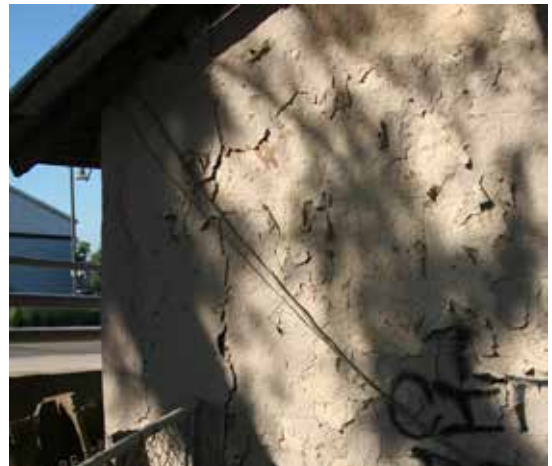
East Wall Crack
