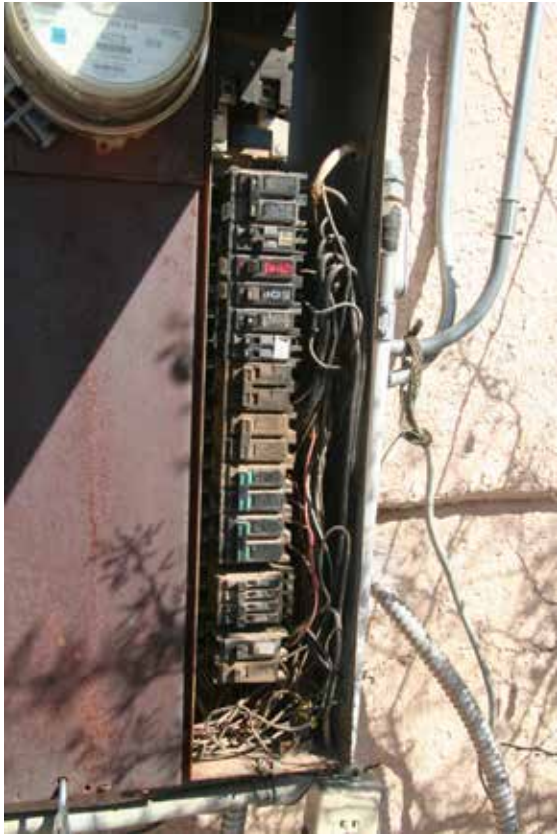
Circuit Breaker Panel
