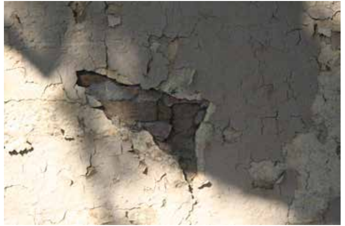
East Wall Damage
