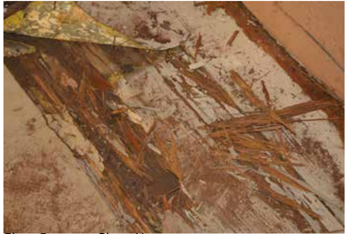
Floor Damage Close Up
