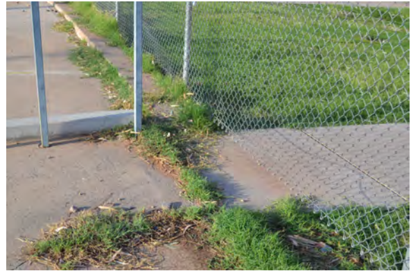
fig. (26) Historic curbing has been removed to allow sidewalk access from Pennysaver site. Photo 2018.
