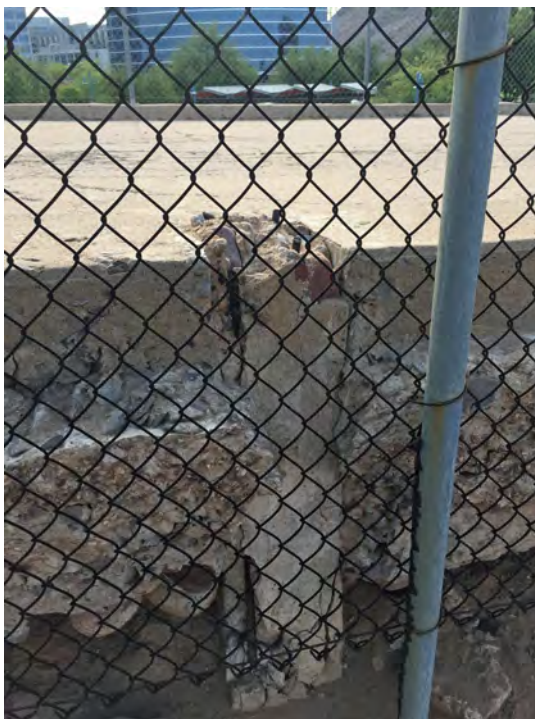
fig. (29) Historic roadbed bollard on west curb showing penetration of roadbed and erosion of roadbed subbase material. Photo 2018.
