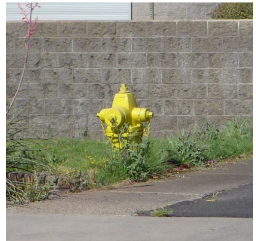
Photo, South River Drive fire hydrant
