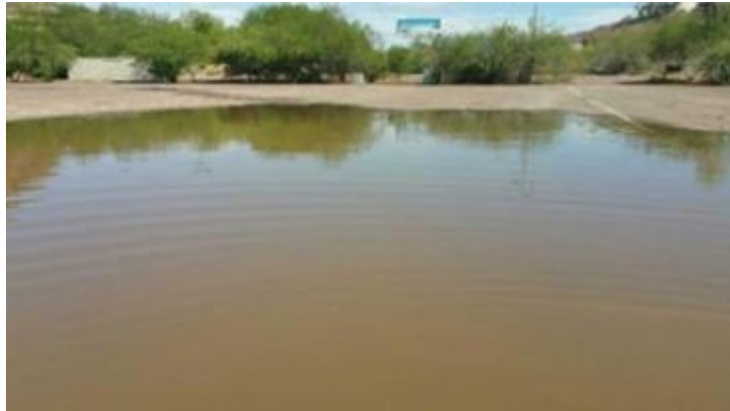
Flooding caused by a clogged inlet
