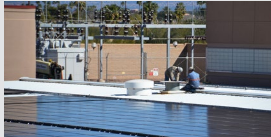
Solar panels on JGM water treatment plant (source: City of Tempe)
