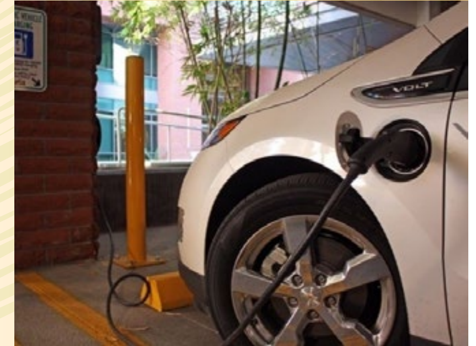
EV charging station at Arizona State University (source: City of Tempe)
