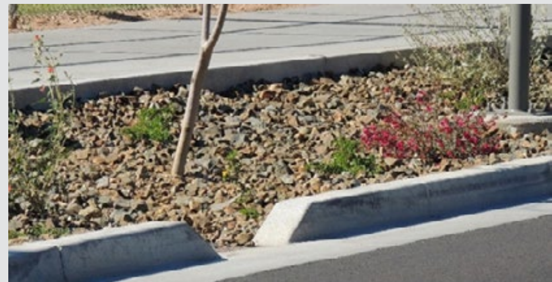
Grated curbs allow stormwater to pass through (source: City of Mesa)
