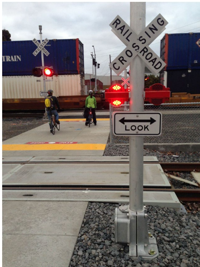
Figure 24 Pedestrian and Bicycle Rail Crossing Signal Example
