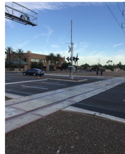
Recently installed UPRR equipment at Broadway Drive
