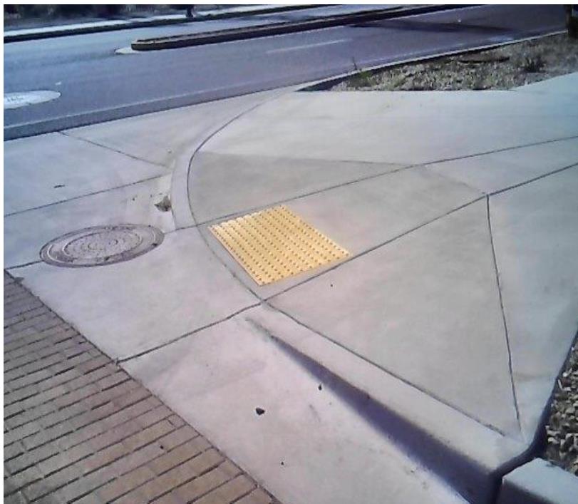
Compliant Perpendicular Ramp
