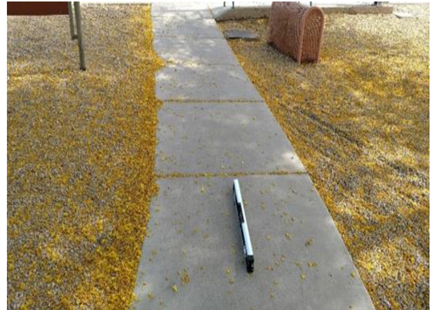
At Creamery Park, the path of travel from the transit stop the Ramada has a non-compliant run slope exceeding 8.33%
