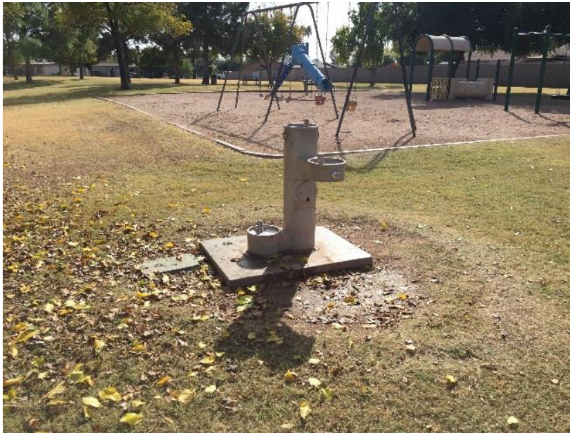
Drinking fountain with no accessible route.
