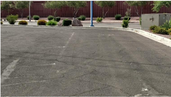
Large parking area for buses/trailers with faded striping
