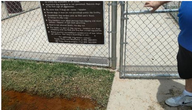
Clark Park dog park gate is missing 18” clear space on the pull side of the gate.
