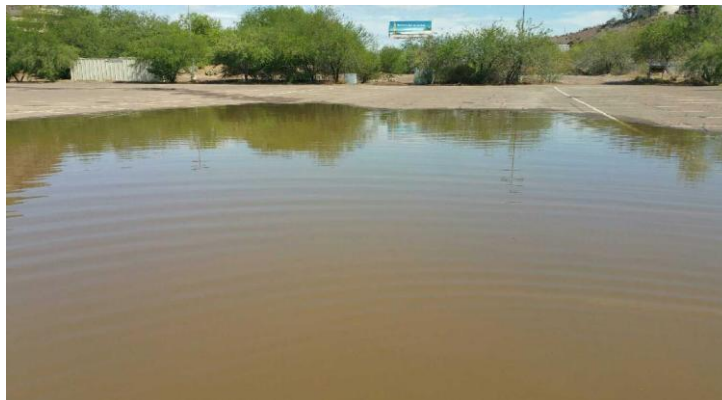
Flooding caused by clogged inlet
