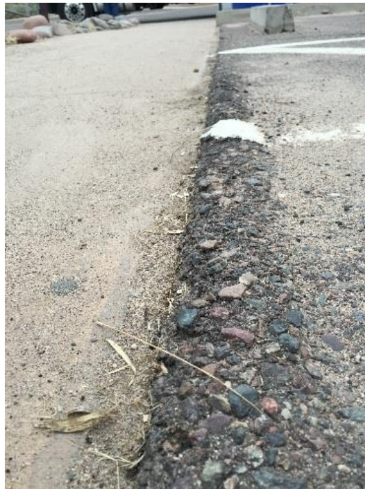
Figure 22: Level change between parking and accessible route
