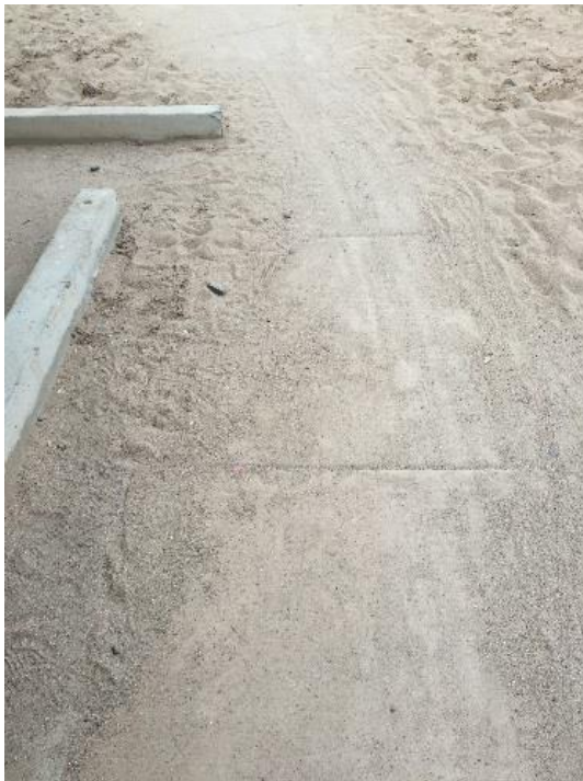
Figure 21: Sand covering accessible route
