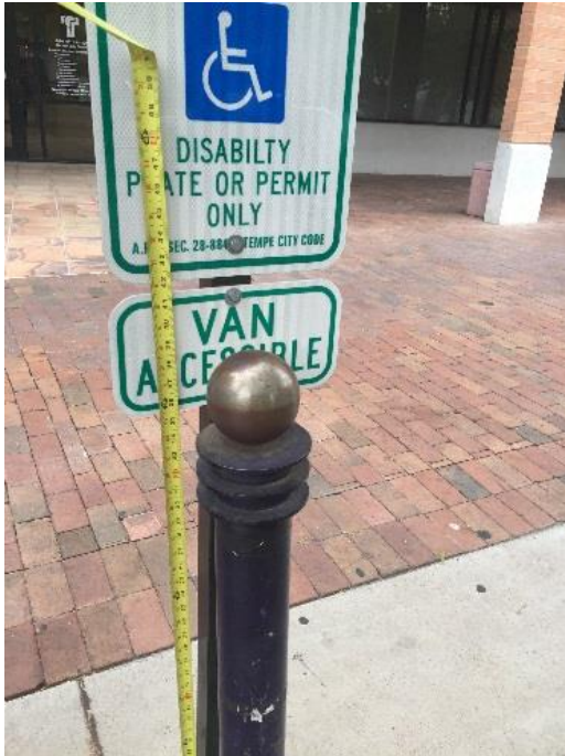
Figure 12: Parking signs too low.
