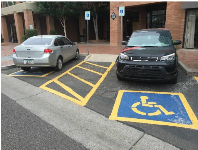
Figure 6: 3 rd St. – Curb ramp within access aisle and 15% slope on curb ramp
