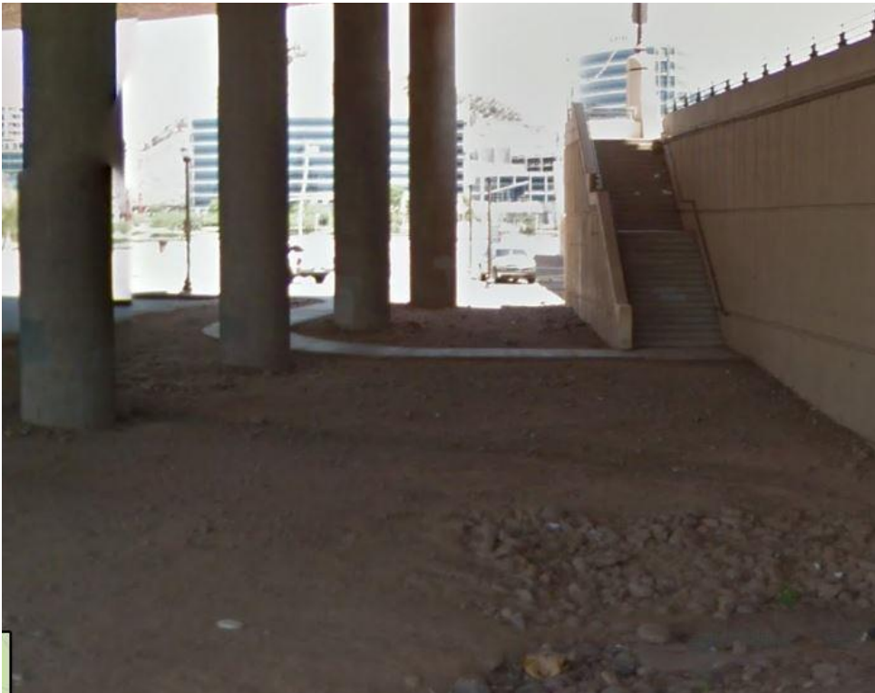
Figure 23: No accessible route from Mill Ave.
