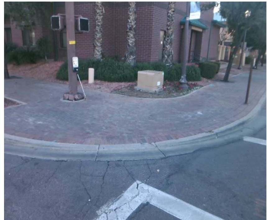
Missing Curb Ramp
