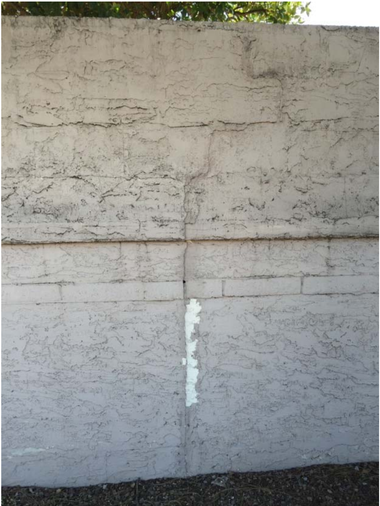
Stucco repair required. Discoloration requires pressure spraying and cleaning.
