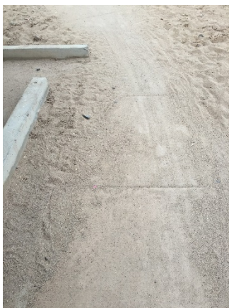
Figure 21: Sand covering accessible route
