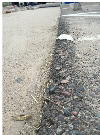
Figure 22: Level change between parking and accessible route
