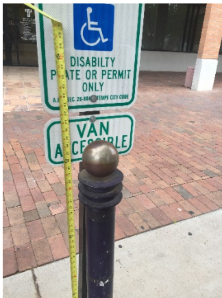
Figure 12: Parking signs too low.
