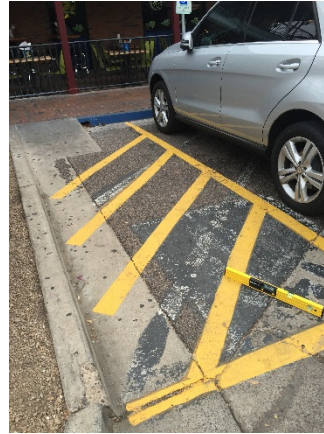
Figure 7: W. 4 th St. – Curb ramp within access aisle
