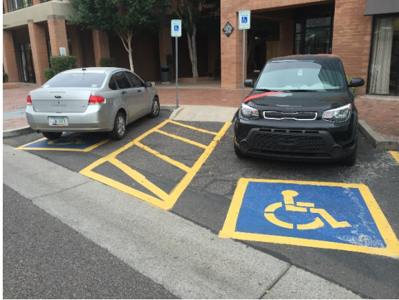
Figure 6: W. 3 rd St. – Curb ramp within access aisle. 15% slope on curb ramp
