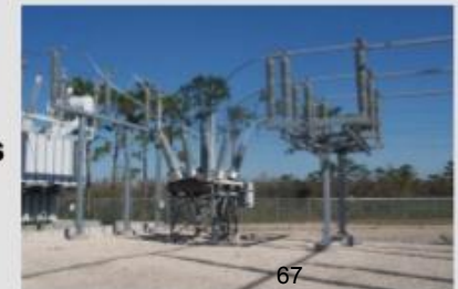
Commuter Rail – Outdoor Substations
