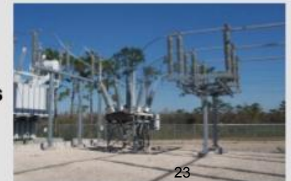
Commuter Rail – Outdoor Substations
