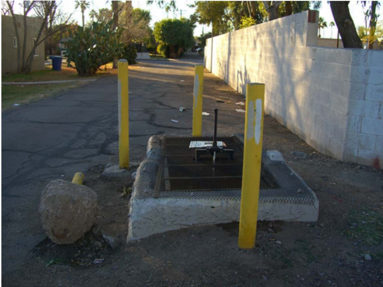
Gate Valve in alley behind Burger King
