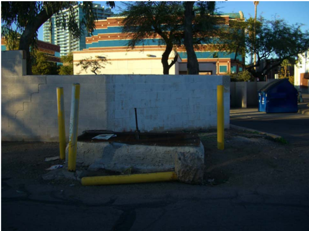
Gate Valve in alley behind Burger King
