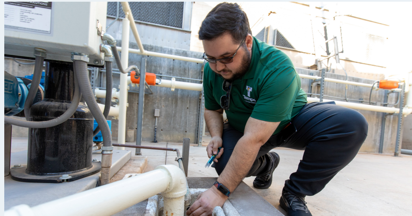
Water conservation program coordinators evaluate infrastructure upgrades for incentive programs, such as the cooling tower rebate, to ensure significant and permanent increases in water use efficiency.
