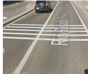
Low rumble strips on the approach to bring awareness
