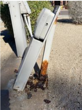
Controllers that need to be replaced
