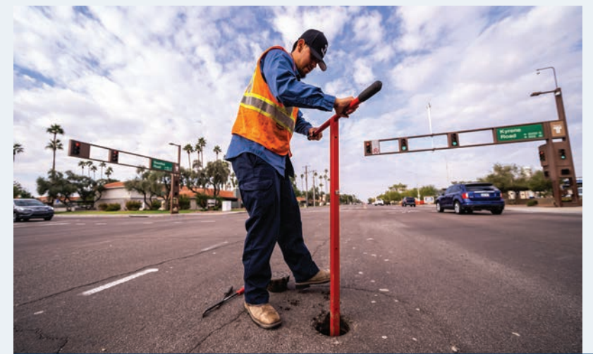
Utility services technicians ensure valves work properly, allowing water to be delivered 24 hours a day and limiting outages to customers during emergencies.
