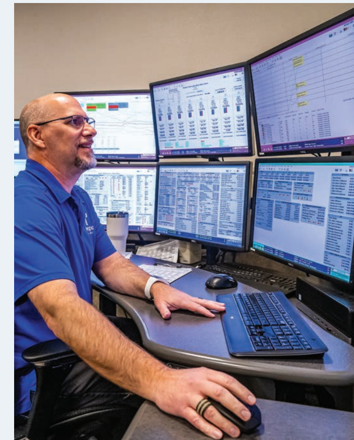
Control center operators monitor Tempe's water treatment and distribution systems to ensure sufficient production and efficient delivery of high-quality drinking water.
