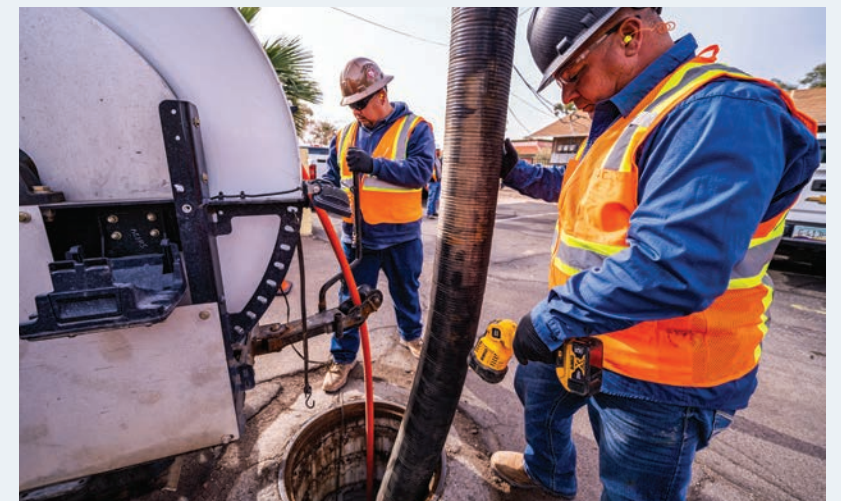
Utility services technicians perform maintenance on the wastewater collection system, preventing sewer stoppages that can pose a risk to health and the environment.
