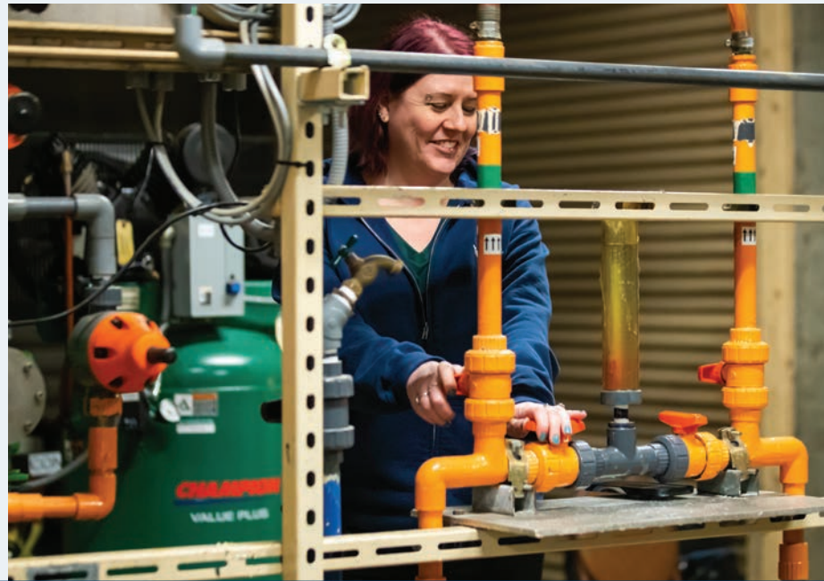
Plant operators oversee the surface water treatment process to ensure the potable water is safe and available for the community's immediate needs.
