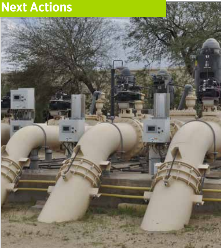
Municipal Utilities water pumps
