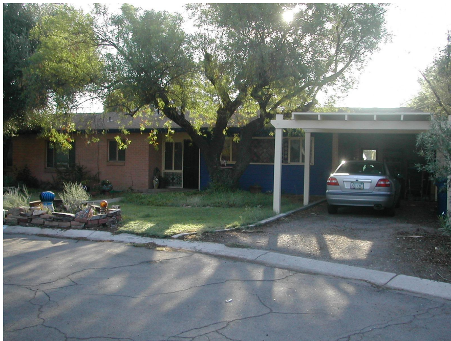
Carport Extension with roof form and material palette inconsistent with original house (Site 241)
