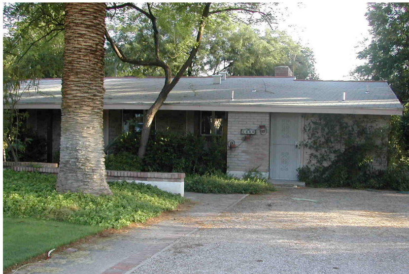
Incompatible Enclosure into Habitable Space with an additional entry door (Site 115)
