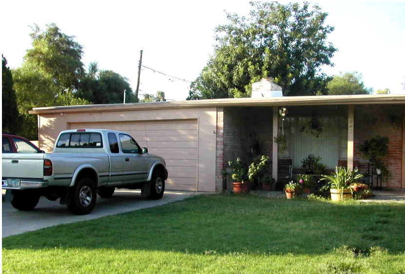
Incompatible Garage Conversion with the addition of a second car bay and incongruous building materials (Site 111)
