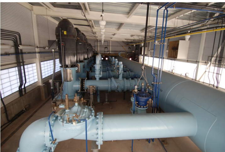
Water pumps at the Martinez WTP
